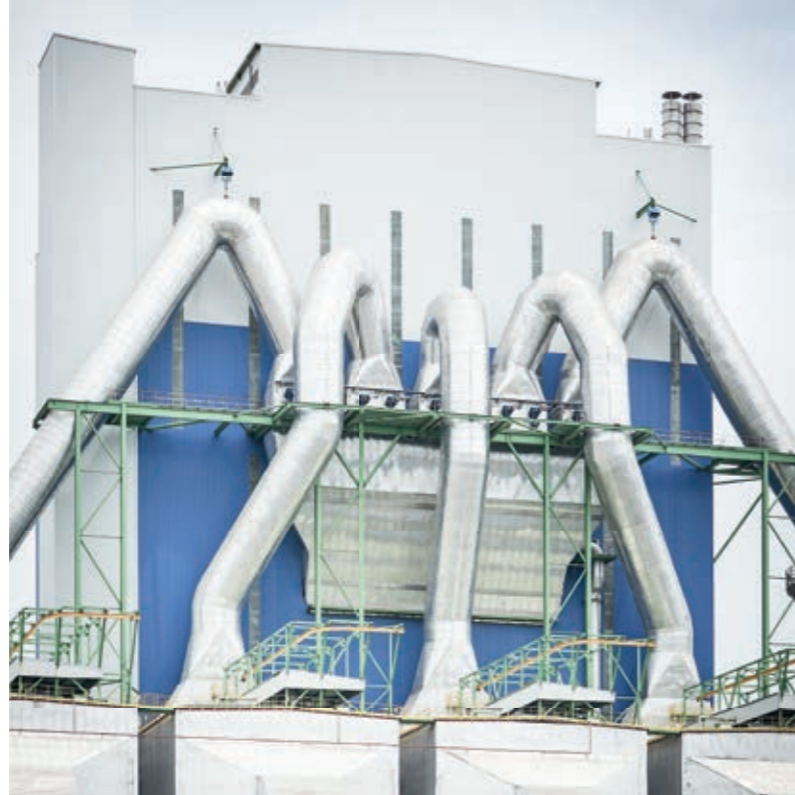
The recovery boiler at OKI is the world's largest boiler today. The unit could easily supply power to a European city of one million inhabitants with an output of 10,000 – 12,000 MWh per day.
