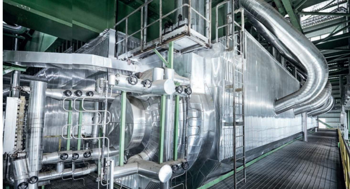
The steam drum in the OKI recovery boiler is the largest in operation today. It weighs 270 tonnes with a length of 23 m.
