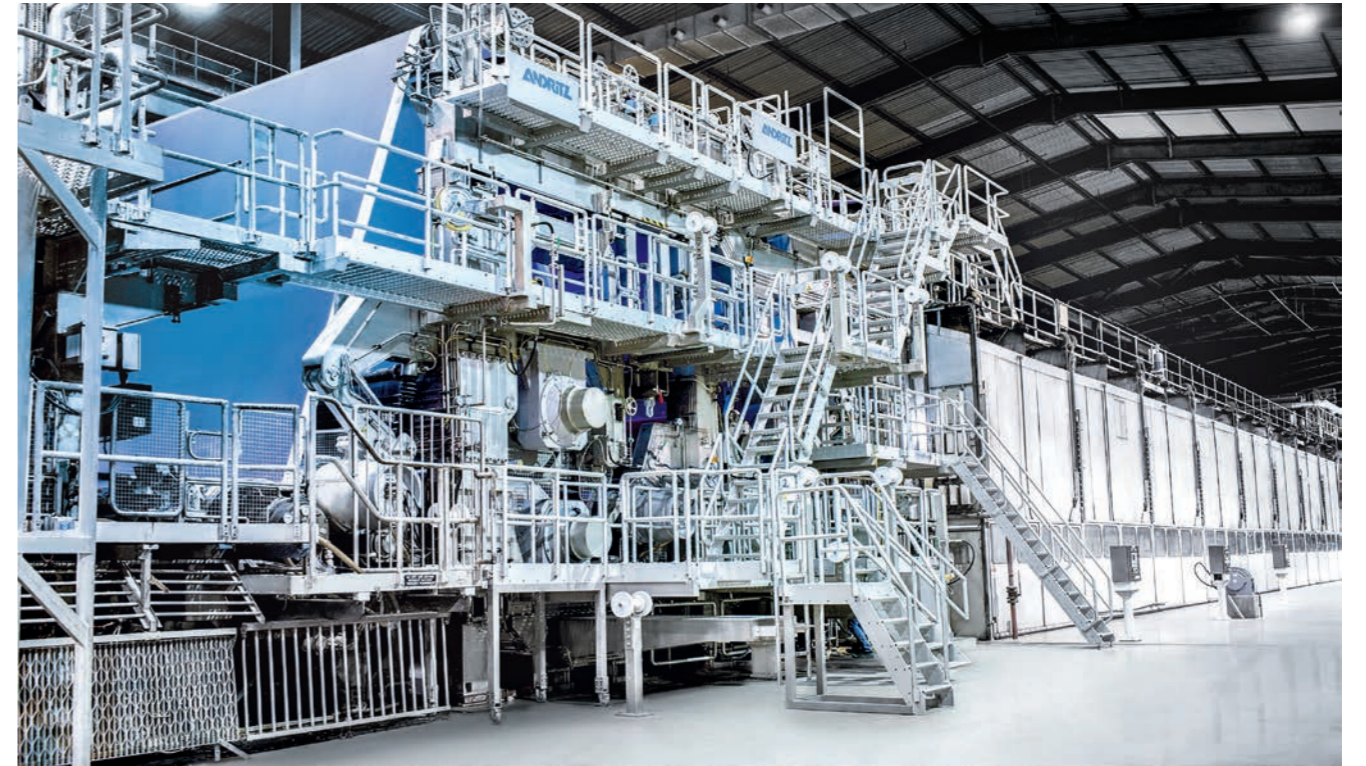
ANDRITZ installed a new press section on Iggesund's BM2, including a long-nip jumbo press with large diameter rolls, an energy-efficient PrimePress X shoe press in the second nip, and a smoothing press. The delivery also included ANDRITZ's state-of-the-art PrimeFeeder vacuum system for ropeless tail threading from the press section to dryer section.
