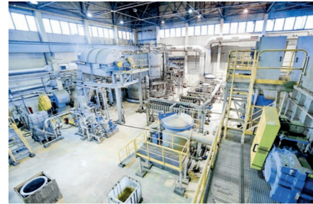
ANDRITZ also delivered a new recycled fiber processing line and machine approach system with a capacity of 800 t/d to bring high-quality stock to PM7's new headbox.
