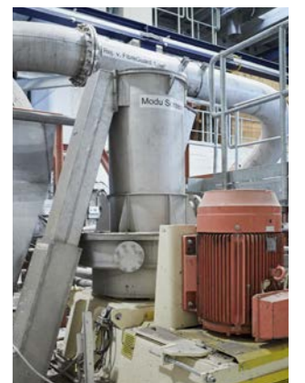
ModuScreens TD tailing screens are part of coarse screening. Efficient washing of fibers is done with a FibreWash Drum – one important part of the detaching system.
