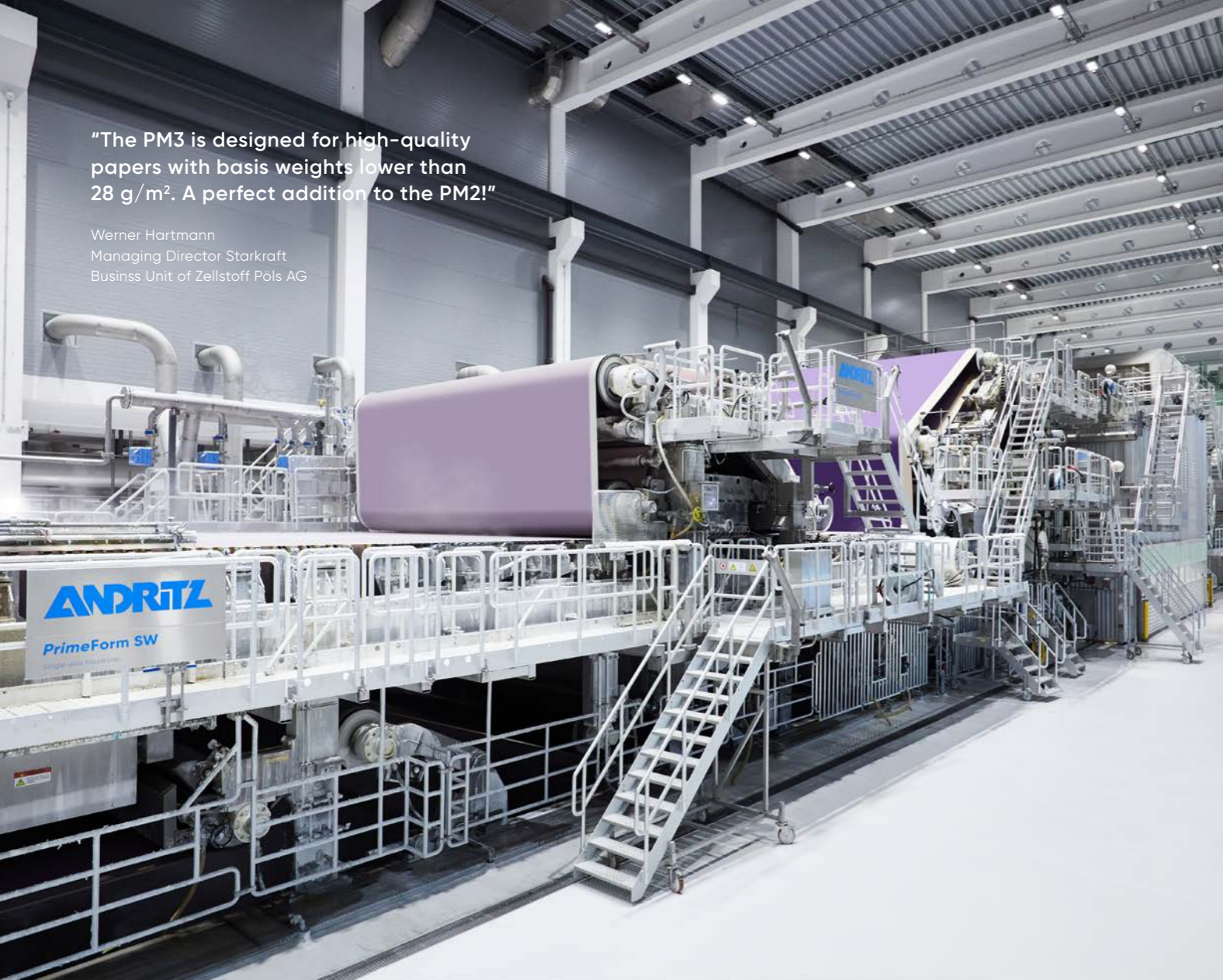
The new PM3: an ANDRITZ solution from the headbox to the reel, including stock preparation, automation and pumps
