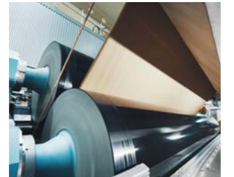
The PrimeFilm film press applies starch simultaneously to both sides of the paper web in order to achieve the desired strength values at the high speed.
