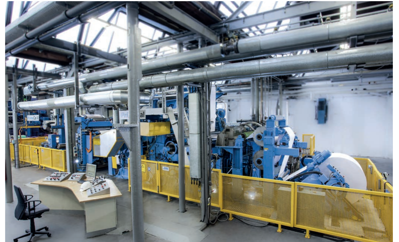
The calender pilot plant at the ANDRITZ Paper Technology Center in Krefeld, Germany
