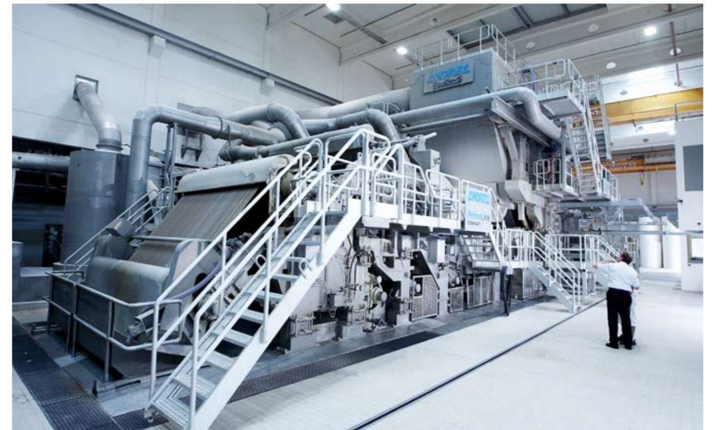
▼▲ The PrimeLineCOMPACT machine (PM6) at Fripa is configured for 30,000 t/a production with a machine speed up to 2000 m/min. The paper width is 2.75 m.
