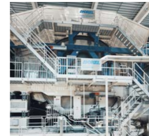
PrimeDry Hood Steam heated MG hood with 190° C temperature. Energy from biomass boiler
