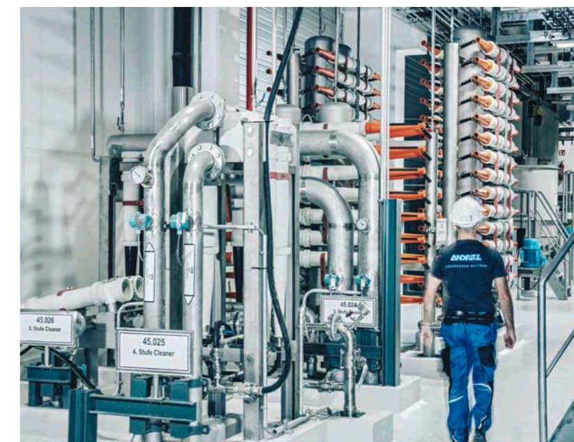
Five-stage cleaner plant for the new PM3
