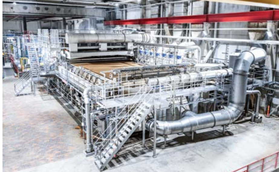
The upgrade project included a rebuild of the complete pulp drying line.
