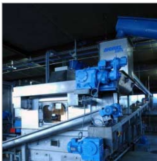
Belt dryer for different sludges in Elgg, Switzerland.
