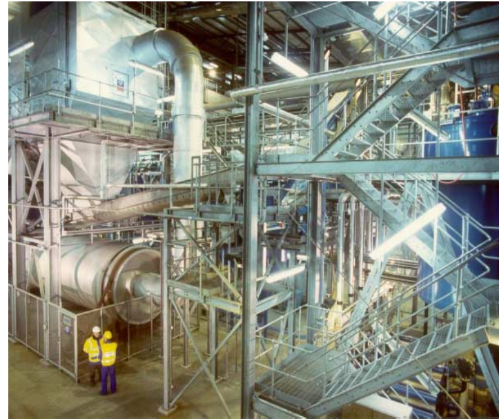
Drum drying plant Bran Sands, UK
