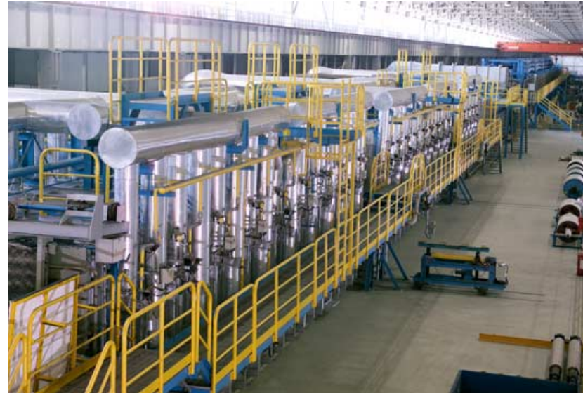
Annealing and pickling line for SKS, China
