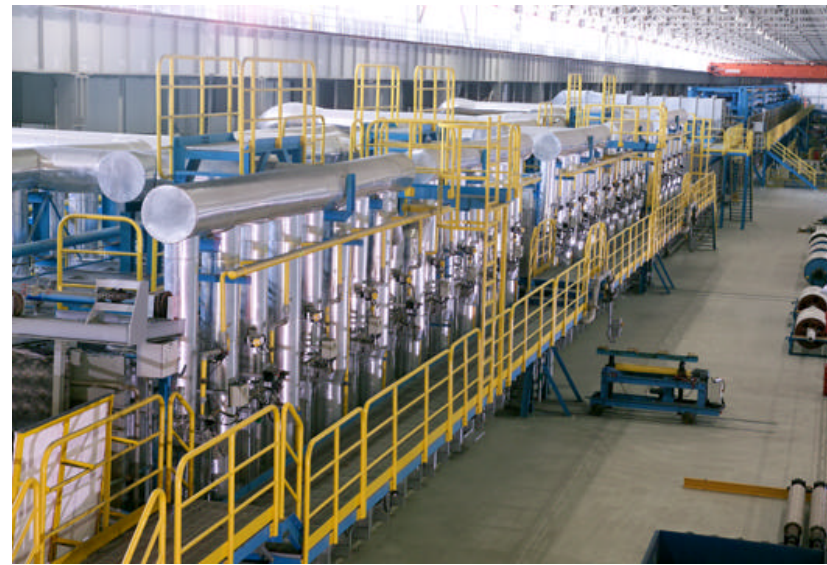
Annealing and pickling line for SKS, China
