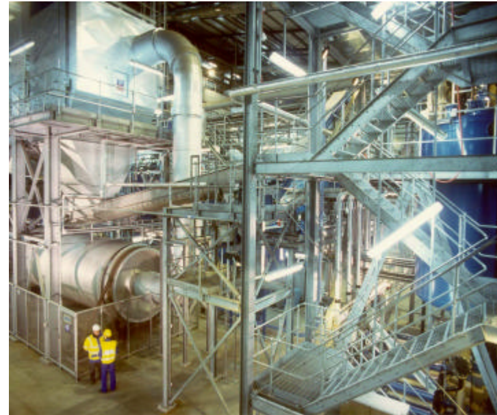
Drum drying plant Bran Sands, UK
