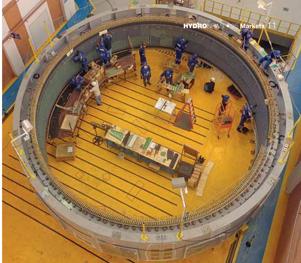
▲ Winding assembly in HPP Cachoeira Dourada
