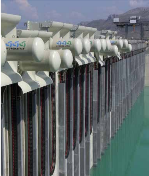
Figure 5: Upstream View of raised TG-Units at Ashta 2
