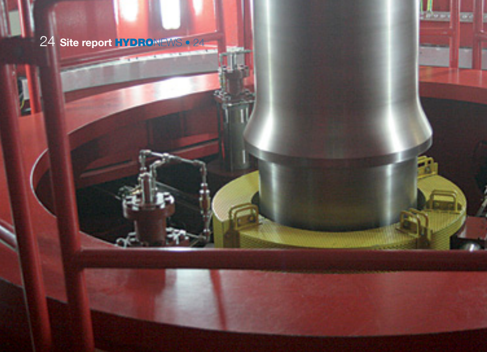
▲ Detail view new turbine unit 3
