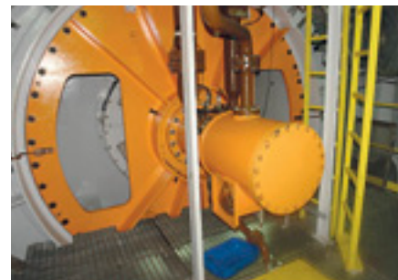
▲ Bulb generator at HPP Santo Antônio
