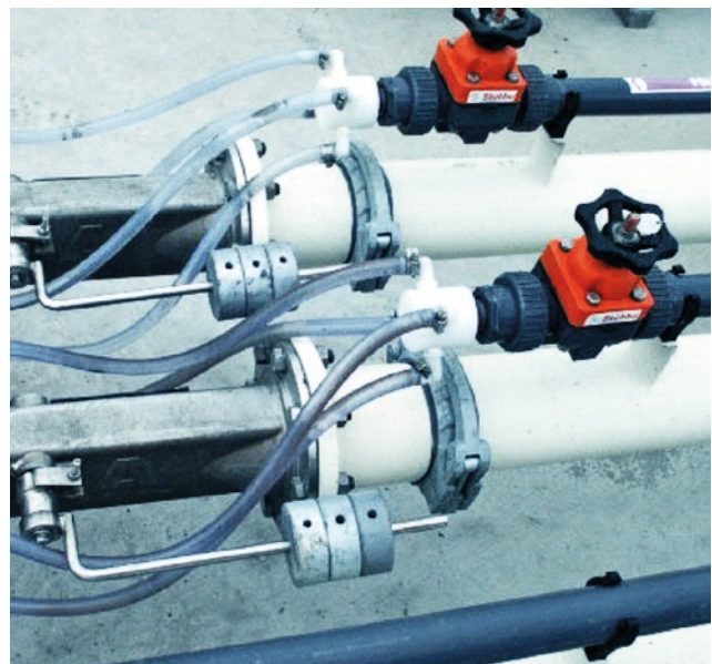
Venturi mixer, inline flocculation system
