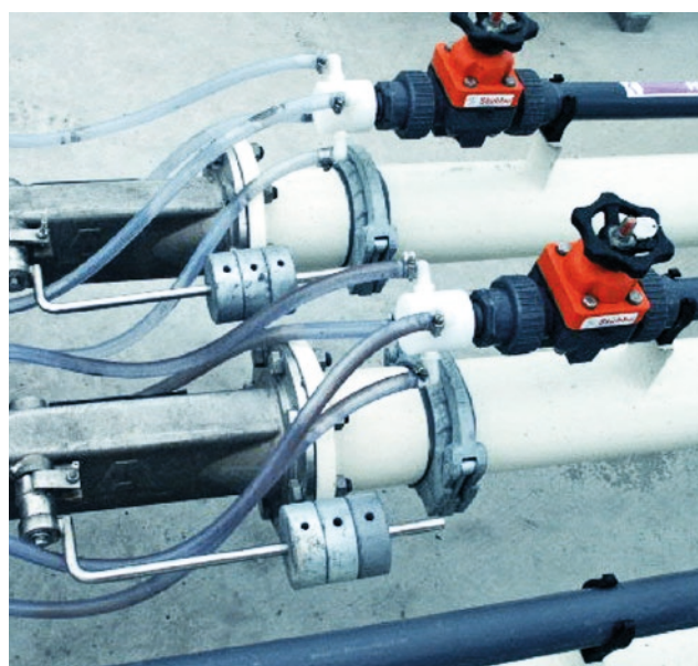
Venturi mixer, inline flocculation system
