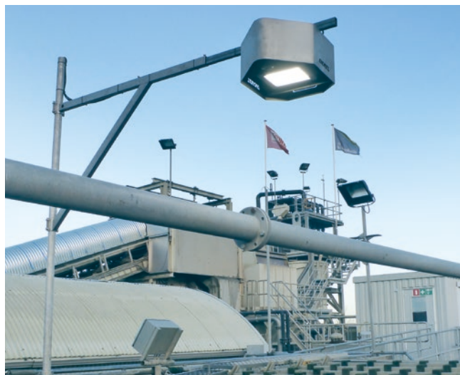
RheoScan installed at a belt filter press
