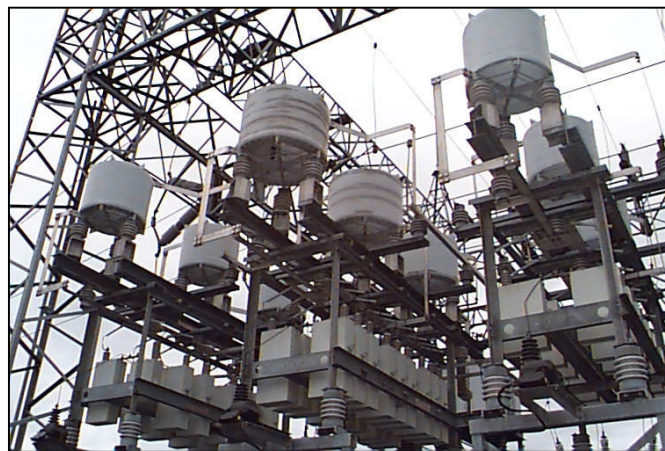
Fig. 1: Line A Harmonic Filter
