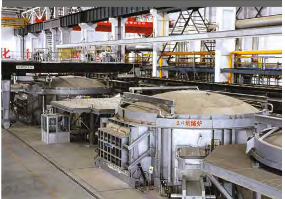
▲ Bricmont-Davy-Swindell melting capacity 120 Mt/hr
