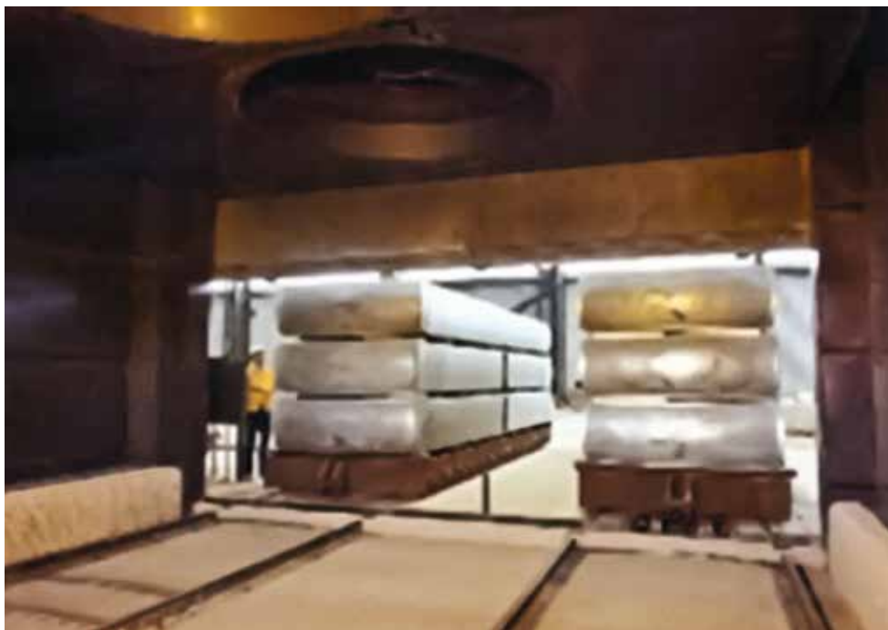
▲ Car bottom ingot heating furnace
