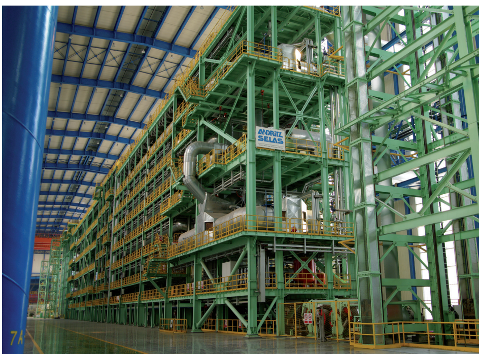
Furnace from entry side
