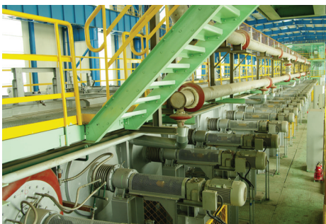
Drive-side furnace rolls
