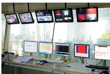
Main control room
