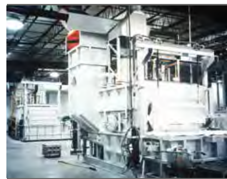
▲ 1,200 kg (2,640 lbs.) per hour radiant roof wet bath reverb
