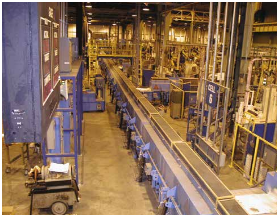
▲ 182 m (600 ft.), 12 station electric launder system
