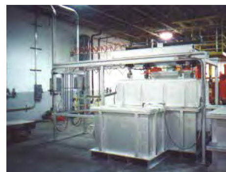
▲ Roll-off lid electric filtration furnace
