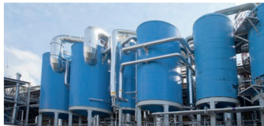
▲ In a unique series of steps, ANDRITZ converted Ružomberok’s two LTV evaporator trains into one plant with falling film technology. Nominal evaporation capacity increased from 470 to 550 t/h.
