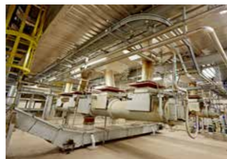
▲ Ash handling system inside the BFB boiler
