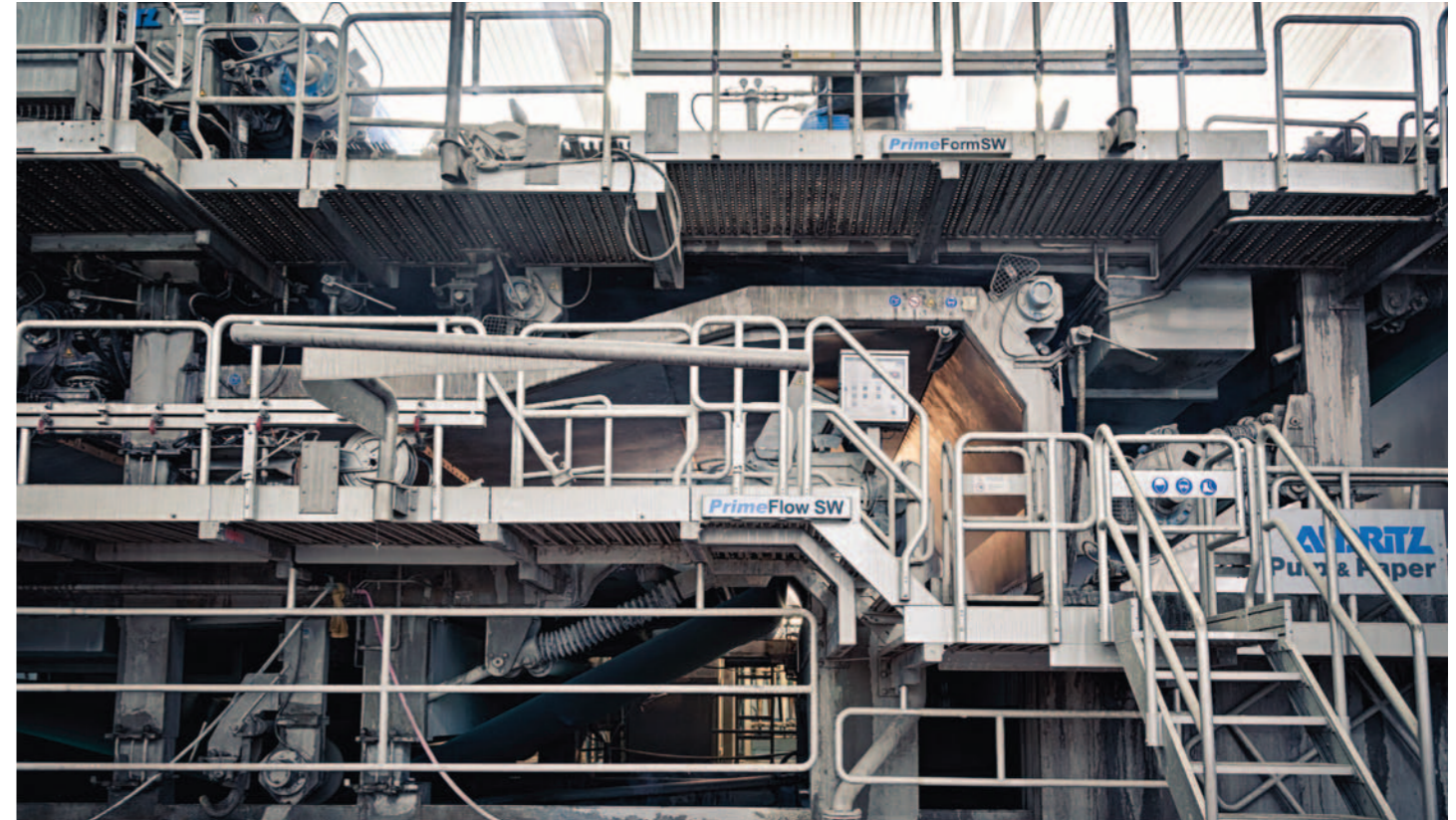
▲ ANDRITZ succeeded in executing the wet end rebuild in only 26 days. The existing cylinder mold formers on PM3 were replaced with a three-layer fourdrinier (PrimeForm SW), which included three new PrimeFlow SW headboxes. The PrimeForm HB is utilized for filler layer dewatering. The existing press section was upgraded with a pick-up roll to allow a closed web run to the press section.
