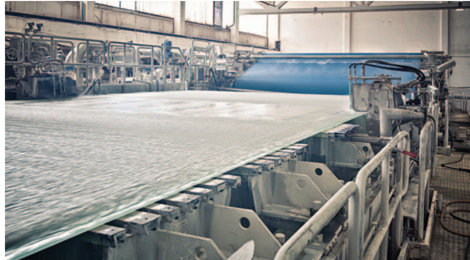
▲ The task was to completely rebuild the wet end on Količevo's PM3 – including a new design hybrid former so it could produce a premium grade of board; in only 10 months from design to start-up.
