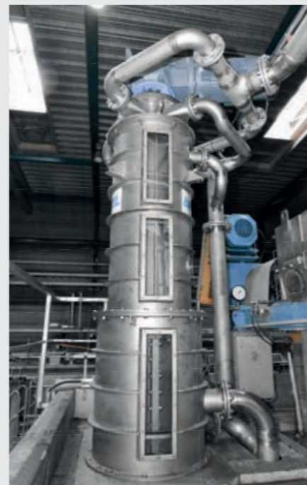
VST in the ANDRITZ pilot plant in Austria.
