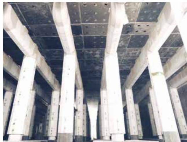
Pre-fabricated insulating shapes mounted at a walking beam furnace
