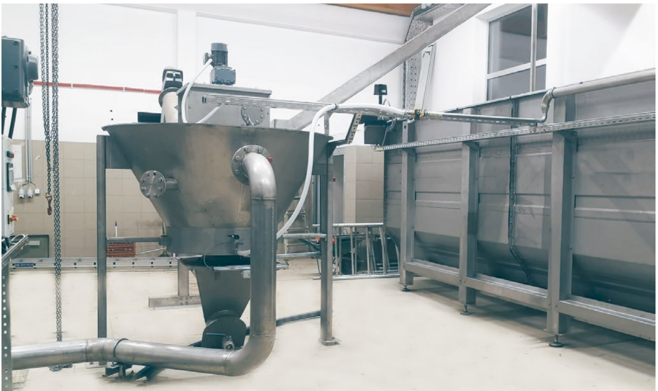
Grit classifier with conveyor to separate sandy materials from wastewater
