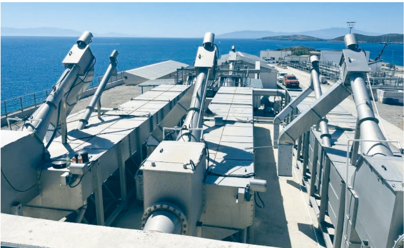
Combo unit, a complete pre-treatment line for screening equipment, grit removal / clarifier and a degreasing
