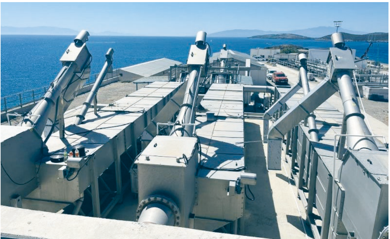
Combo unit, a complete pre-treatment line for screening equipment, grit removal / clarifier and a degreasing
