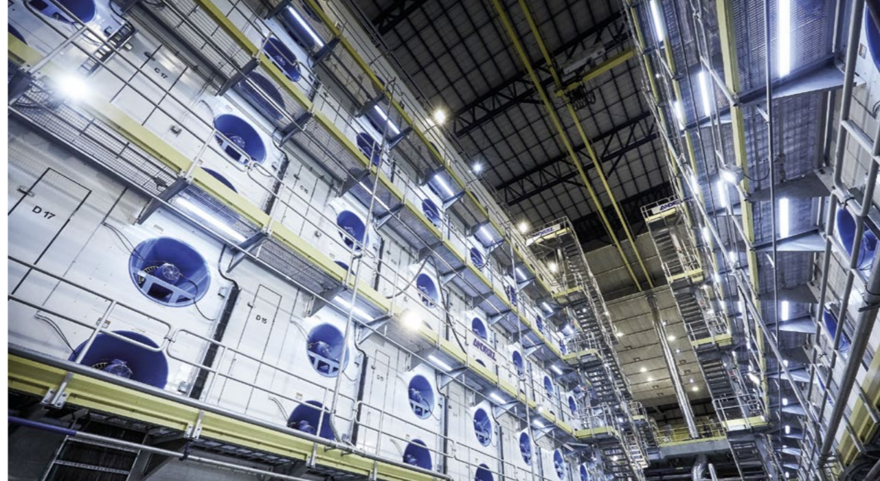
The pulp drying plant is designed for a specific plant capacity of more than 390 tonnes per day and meter of working width, which has been very well-proven for ANDRITZ pulp drying plants all over the world.
