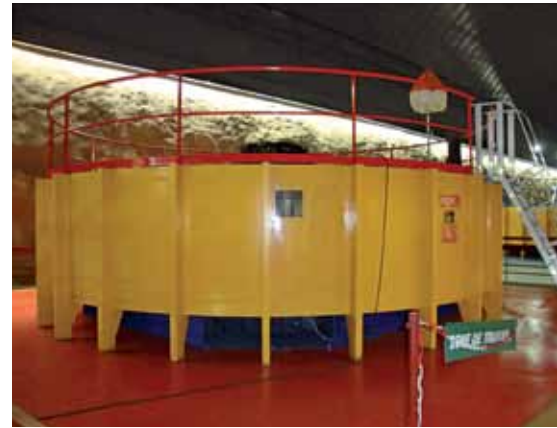
▲ Unit 2 of HPP Revin
