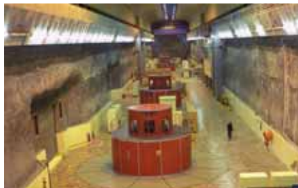
Turbine hall in Drakensberg pumped storage power plant
