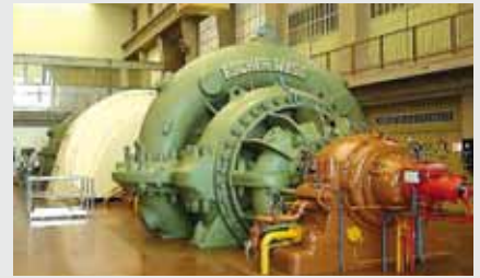
Machine room with pumped storage unit 1
