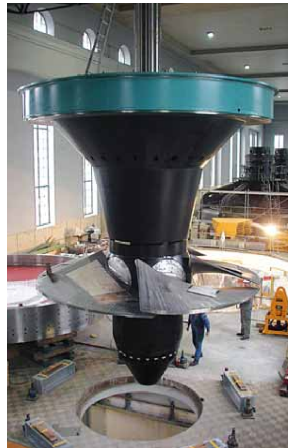
New Kaplan runner on the erection bay
