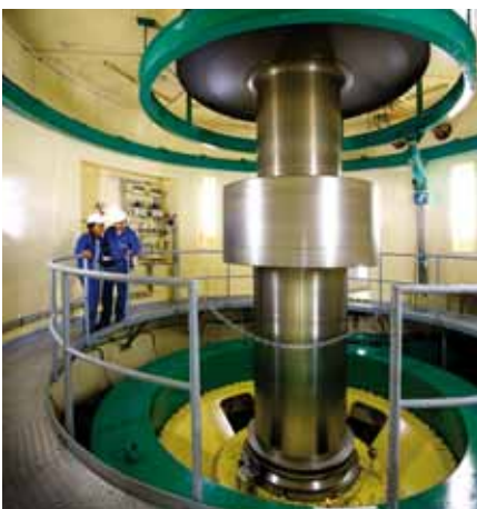
Palmiet turbine shaft
