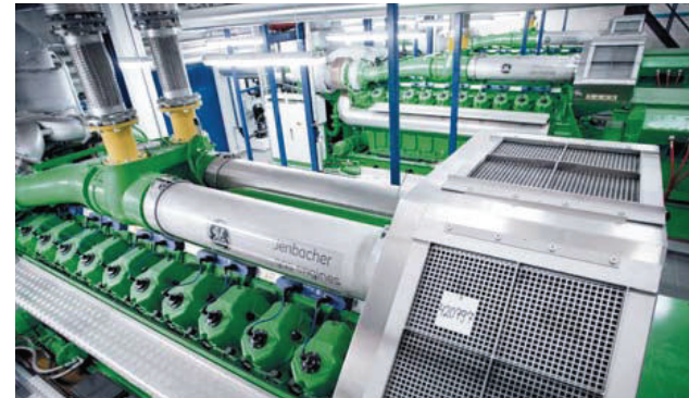
▲ The engine room: three reciprocating engines operate on the biomass-derived fuel from the ANDRITZ Carbona technology.
