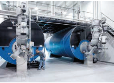
▲ Two gas boilers at the plant can also utilize the product gas from the gasifier to produce additional district heating.
