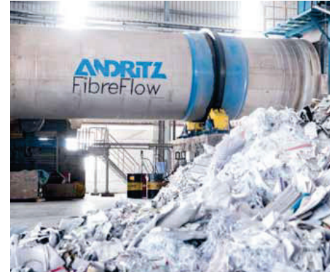
▲ The FibreFlow drum pulper is considered a core technology in the DIP line by TNPL management. It disintegrates the secondary fibers without harming them, while large contaminants are removed intact.
