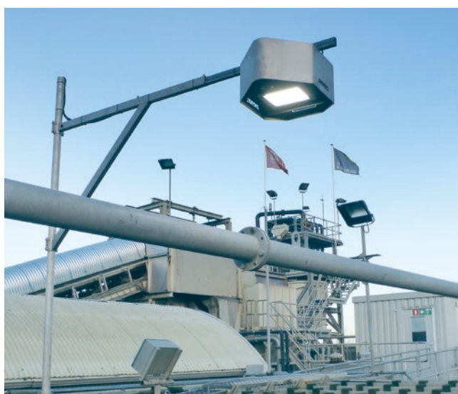
RheoScan installed at a belt filter press
