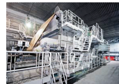
▲ The PrimeForm TW is smoothing production because PM4 is now less affected by variations in the furnish or by operator actions.
