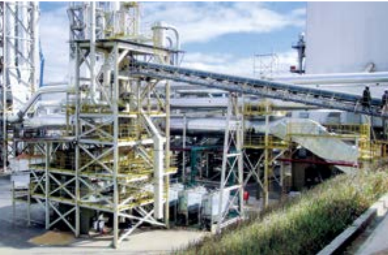
ANDRITZ supplied the chip screening and washing technology seen here.
