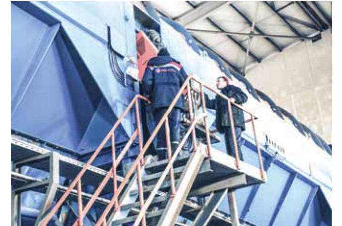
The debarking unit operates around the clock. ANDRITZ trained all operators to run the equipment, which requires only scheduled maintenance at pre-determined intervals.
