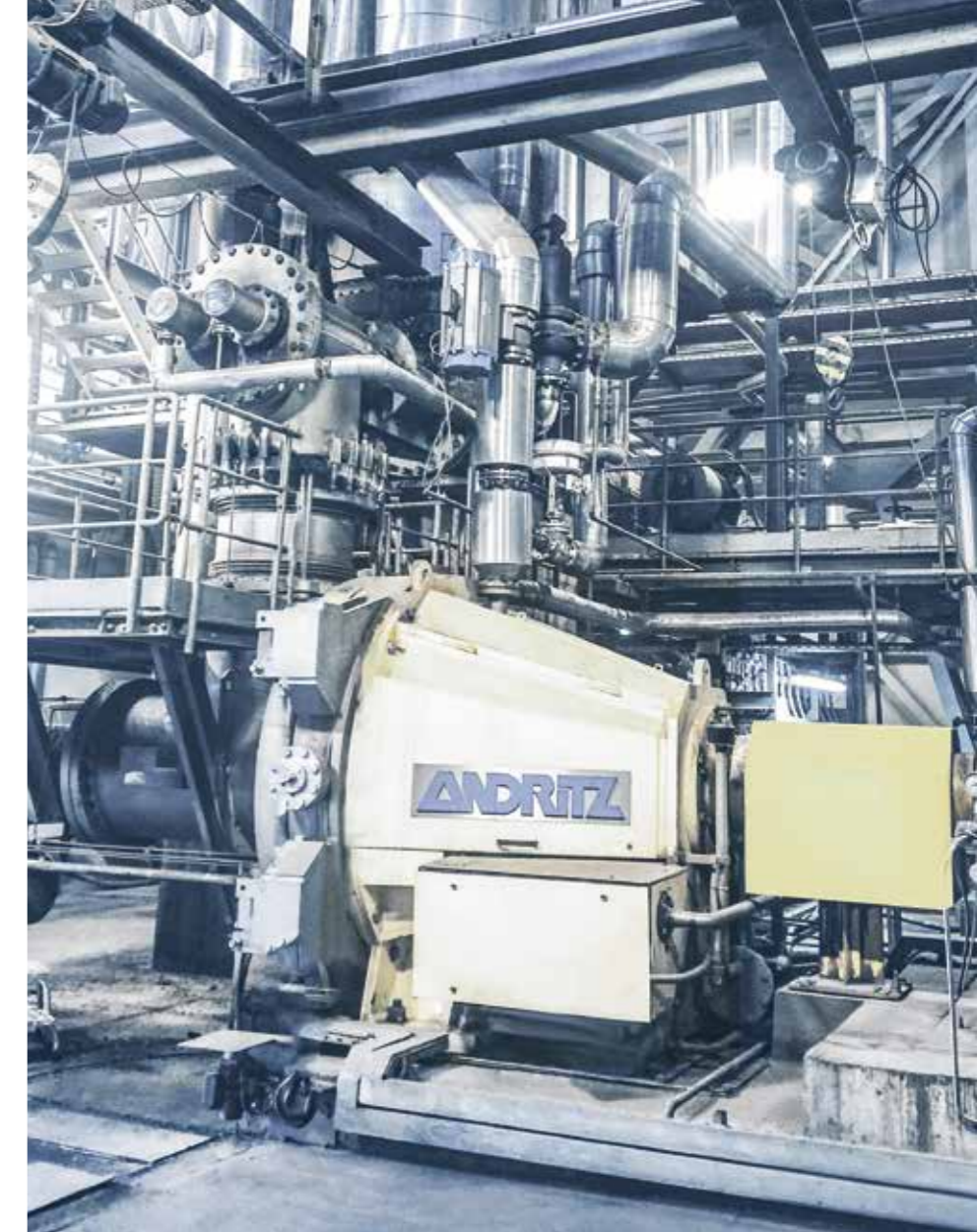
The ANDRITZ pressurized refiner for line 2: This line was purchased and relocated to the site, producing high-quality fiber for the Dieffenbacher press line. An ANDRITZ ribbon feeder precedes the refiner, which operates at constant high speed and ensures that steam from the refining process flows back to the digester.
