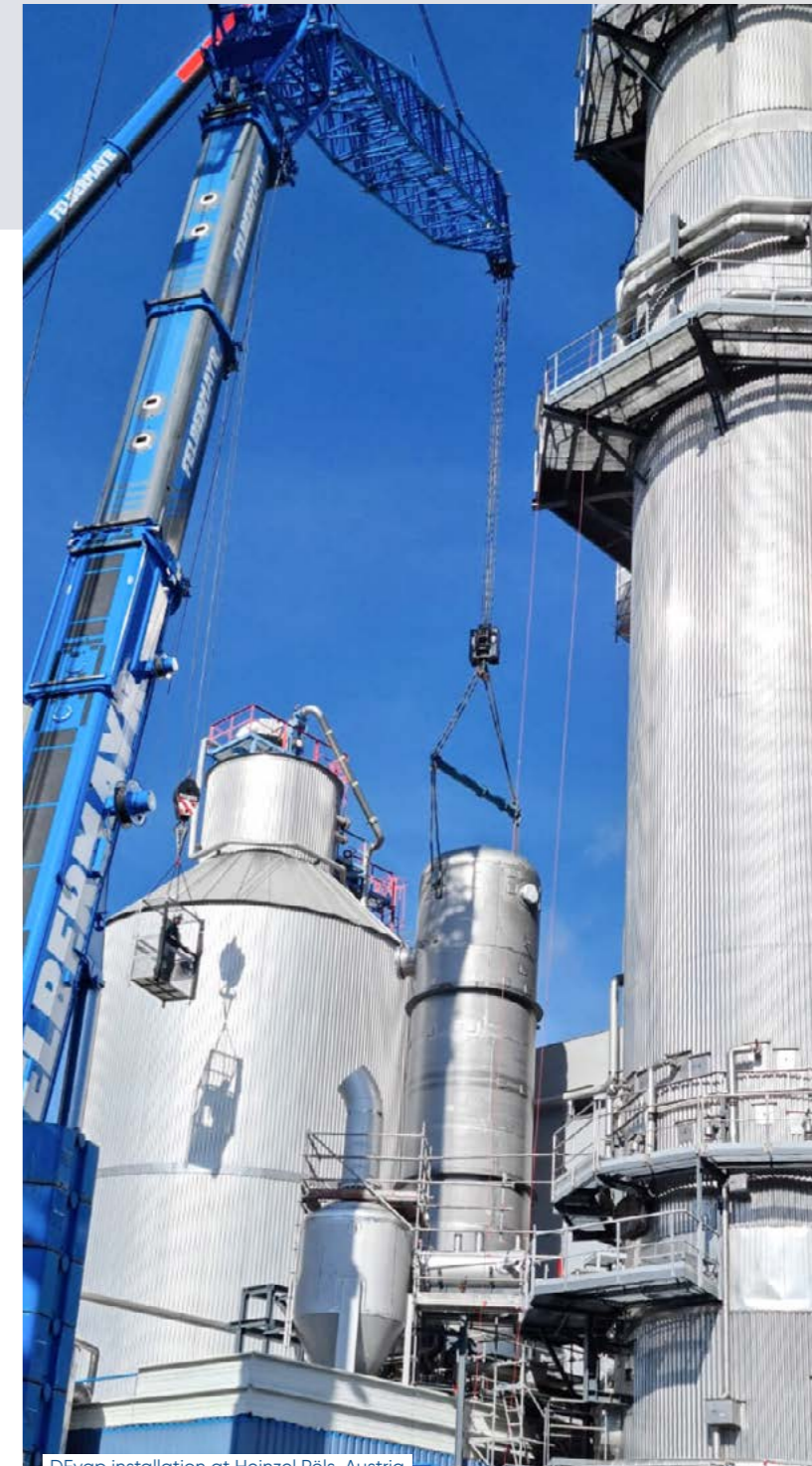
DEvap installation at Heinzl Pöls, Austria
