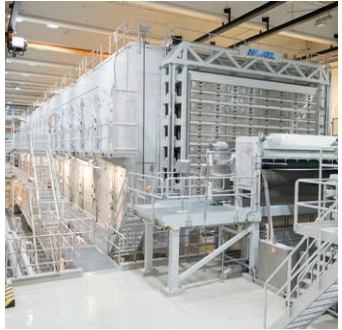
▲ Airborne sheet dryer and cutter/layboy in the new drying plant.
