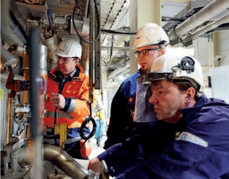
▲ In addition to delivering the recovery boiler when the mill was built, ANDRITZ has remained involved by providing services to improve the boiler's performance even further without major upgrades. Examining systems in the boiler are (l to r): Jan Peter Daum, Recovery Manager at Zellstoff Stendal; Pertti Immonen, ANDRITZ Service Engineer; and P. Raymann of Zellstoff Stendal.
