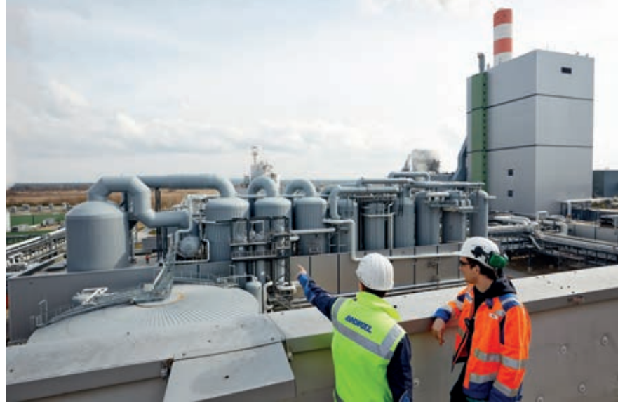
▲ To remove bottlenecks and upgrade the evaporation plant, ANDRITZ delivered new equipment on a tight deadline. The 20% increase in evaporation capacity also allows the recovery boiler to burn higher solids black liquor.
