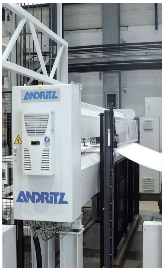
ANDRITZ Scan-X gauge entire view
