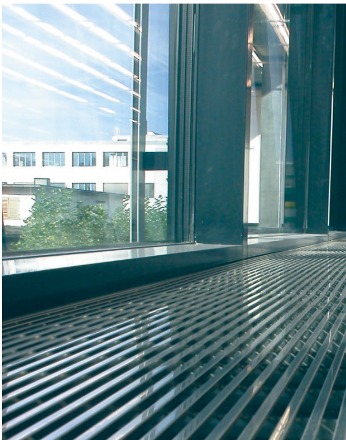
Ventilation floor grille
