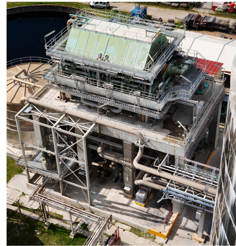
The improvements in brownstock washing came from the relocation of the wash press and replacing six filter washers with just one three-stage DD-Washer.
