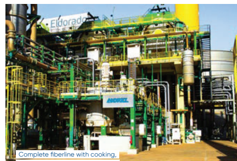
Complete fiberline with cooking, washing, and bleaching systems
