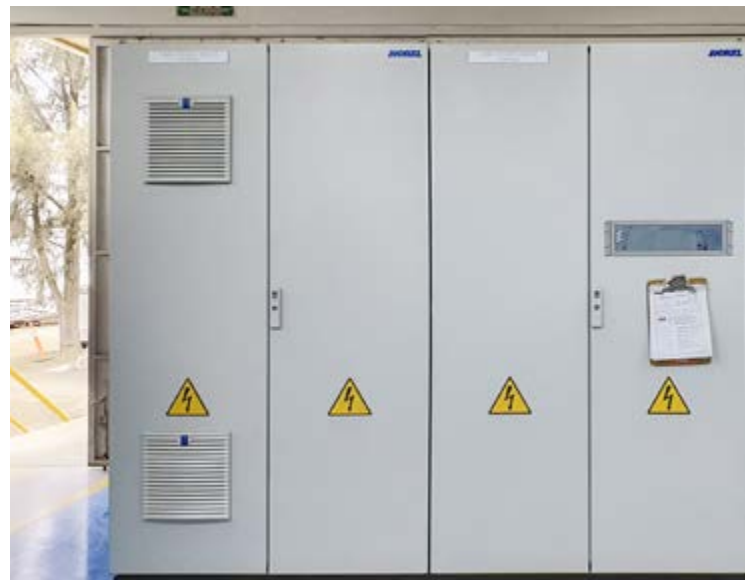
Electric cubicles at Mazatepec hydropower plant
