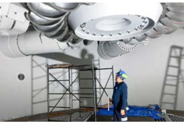
Pelton runner at Zimapan hydropower plant
