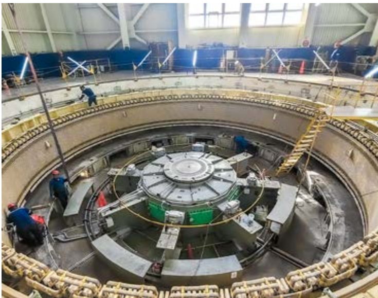
Combined bearing, Unit 1, La Villita hydropower plant
