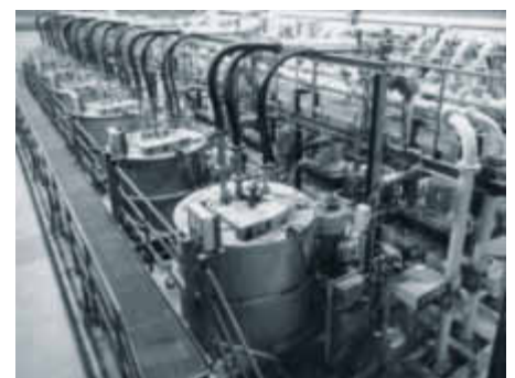
Installation with 42 gypsum centrifuges
